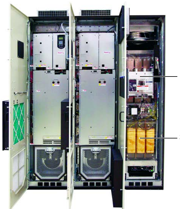
Input power landed behind circuit breaker, which is accessed by extracting rollout
